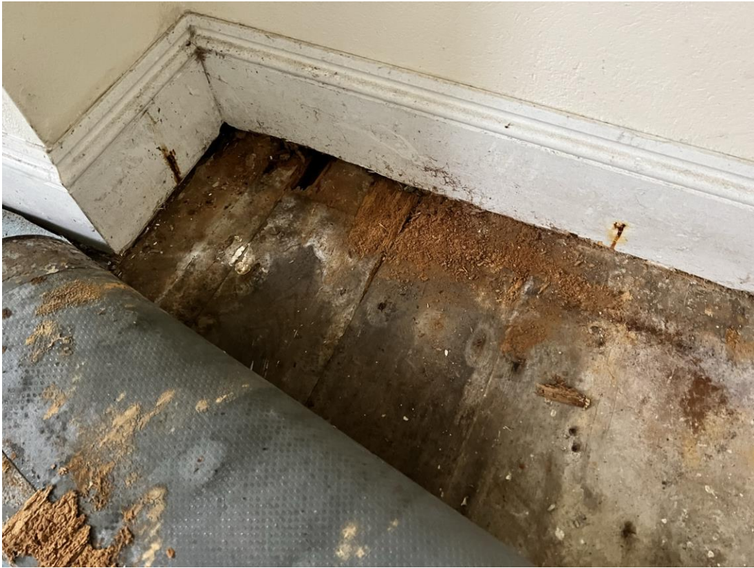
Figure 7 - Rotten floor boards to west end of kitchen.
