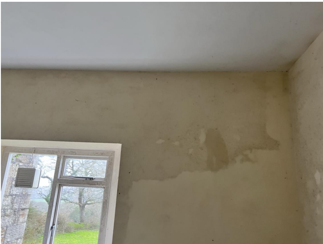
Figure 8 - Significant damp staining to tops of kitchen walls.
