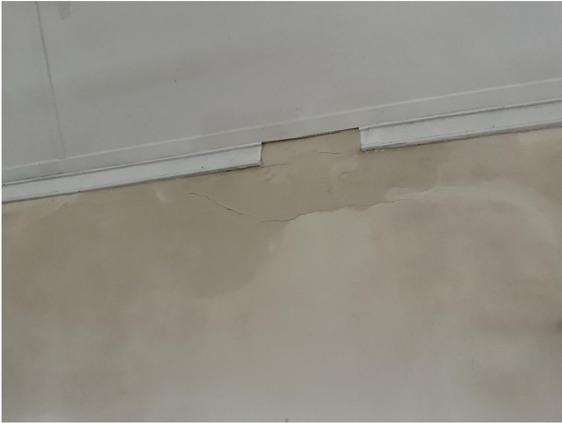
Figure 5 - Damp issues and cracking around base of north chimney.
