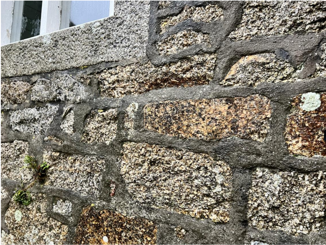
Figure 1 – Cement pointing noted in multiple locations.
