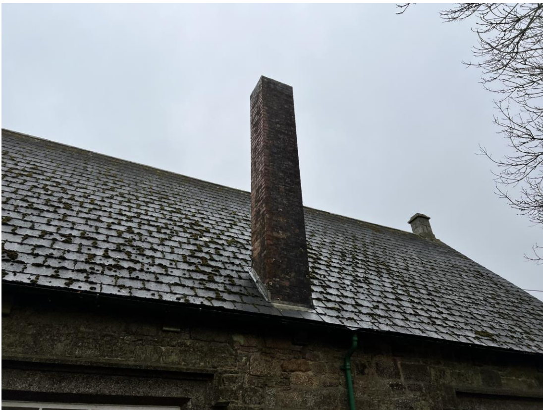
Figure 2 – Roof coming to end of natural life. Very high chimney to north side of building.
