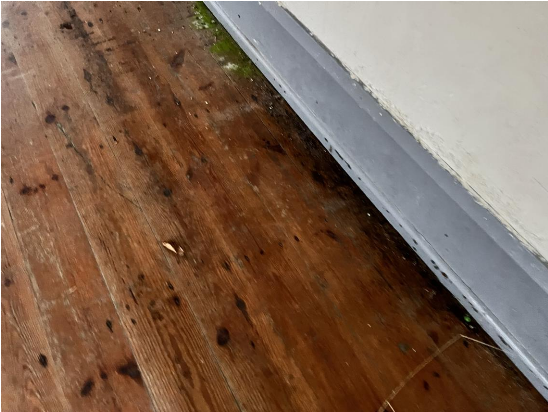
Figure 6 - Rot to floor around centre of south side of main hall.
