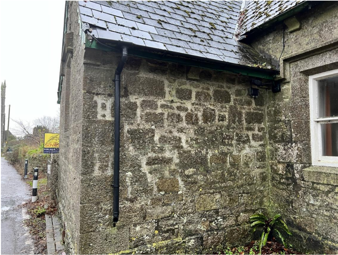
Figure 3 – Evidence of historic repairs and possible movement to porch area.
